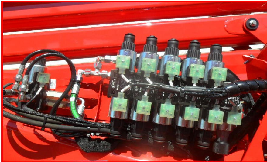
Picture 15: emergency workbench with the main hydraulic distributor.
