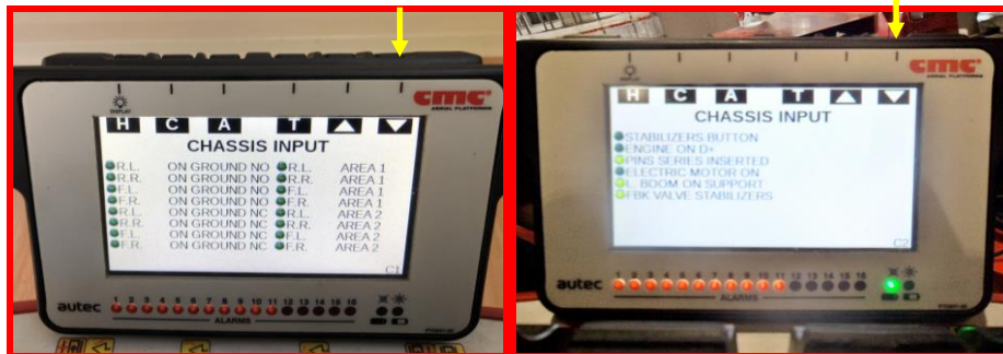
Picture 22: Chassis C1-C2 screens.
