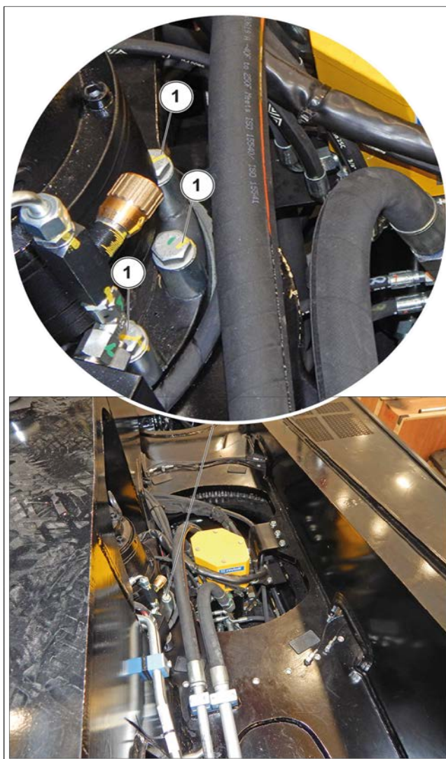
Figure 166: Rotation reducer fixing screw tightening check
